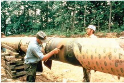
Pipe surface is wire brushed to remove loose scale, rust and dirt.
