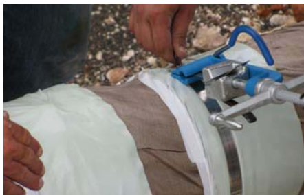
Last wrap of Double-Faced Adhesive with release paper not removed, banding begun.
