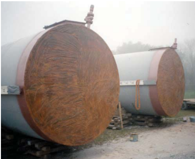
Temcoat 3000 applied to pipe surface. It will then be wrapped with Poly-Ply, Guard-Wrap® or Wax-Tape®.
