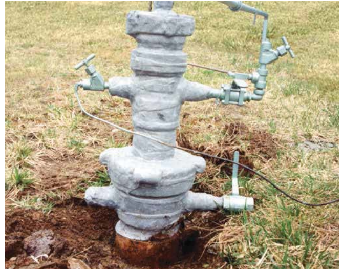
#2A Wax-Tape (aluminum pigmented) easily applied to a difficult-to-protect wellhead. Note the complete conformity to the irregular surfaces.
